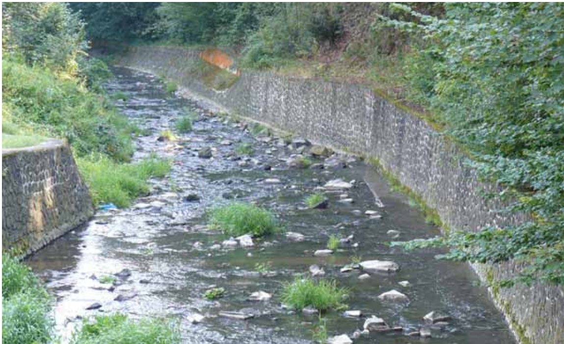
Fig. 3.7. Technical stream regulation that transforms a positive landscape element into a migration barrier.
