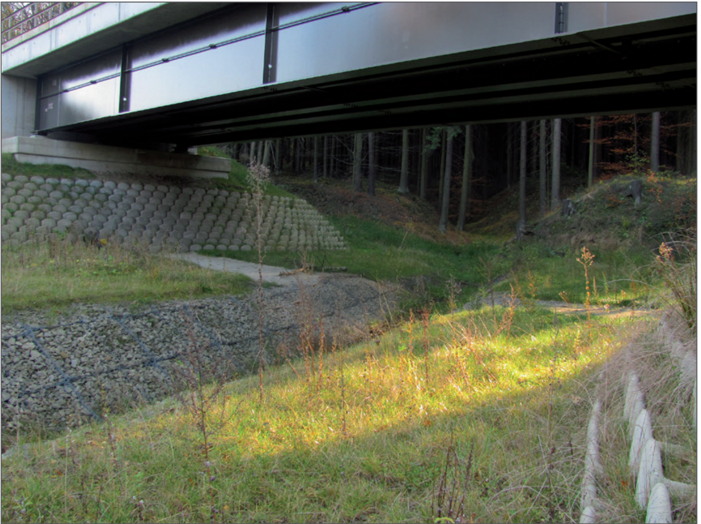
Fig. 2: New underpass under the international railway track no. 320 in the axis of the Jablunkov corridor. Photo by T. Krajča.
